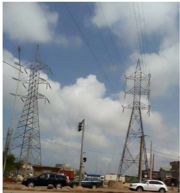
Figure 16: High voltage transmission line L220 of the Electrical Community of Benin (CEB)
